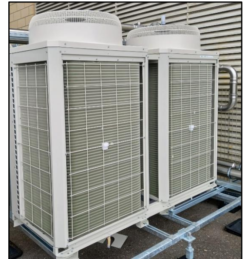
Heat pumps at Exe Valley Leisure Centre
